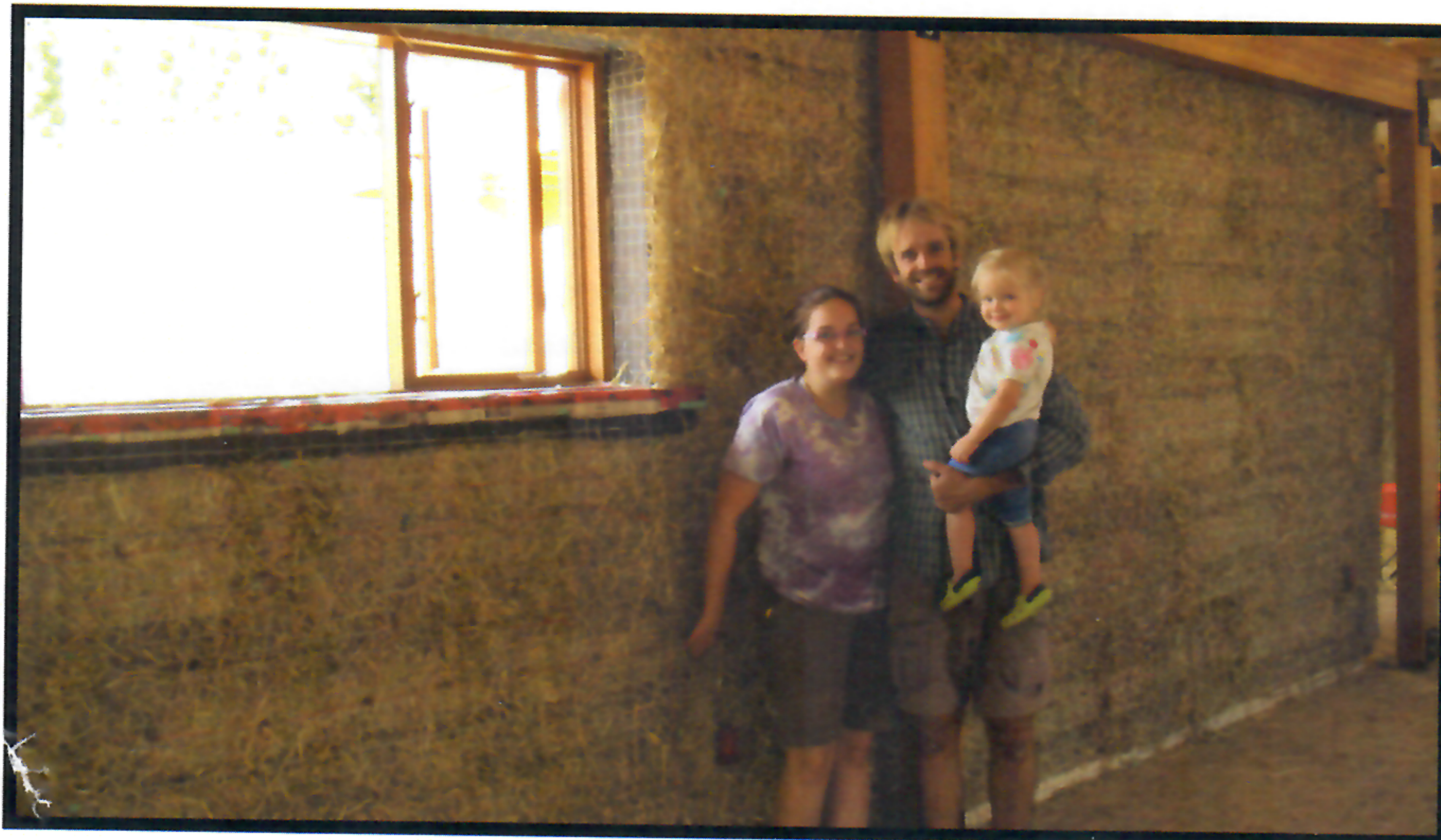
Local Westbank residents Lisa Paynter, her husband Pip Akins and their daughter Eloise sidle up beside one of their newly-built straw bale walls.
